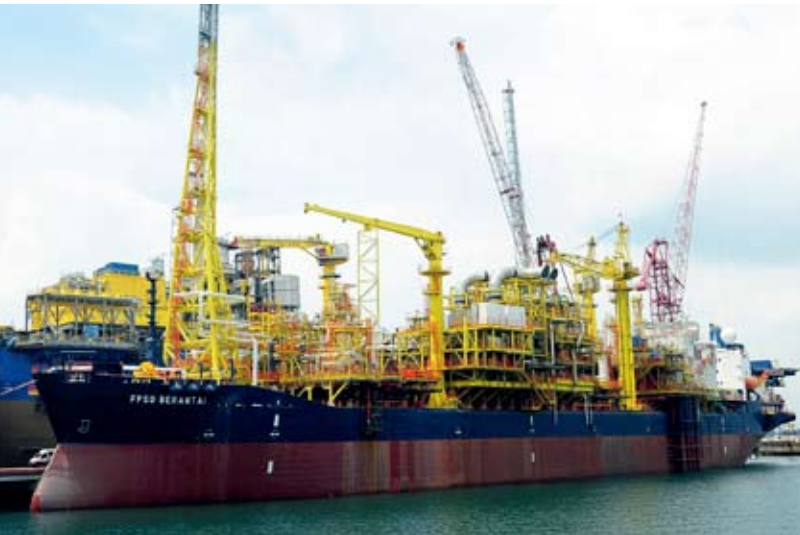
Steady progress on FPSO Berantai, the first FPSO conversion project between Keppel Shipyard and Petrofac
